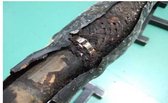
Fig 4. Cable joint failure (Cablejoints.co.uk)
