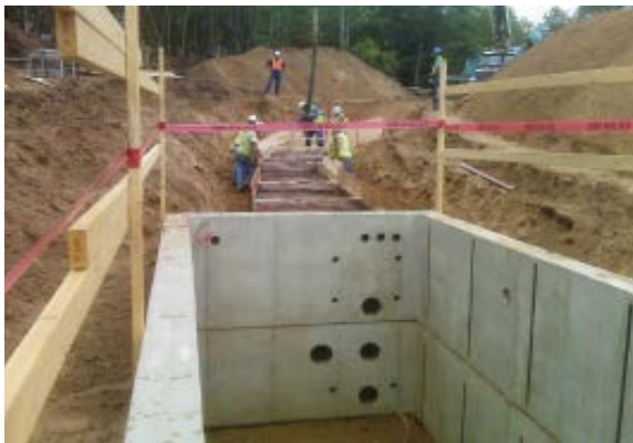
Fig 3. Underground vault (Xcel Energy)
