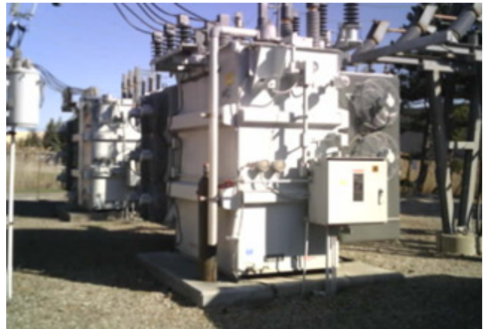
Figure 2 - Visual image of the transformer recorded with the IM500 daily snapshot.
