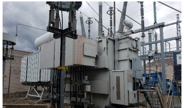
Figure 1 - Low side connections on this transformer are not easily accessible
