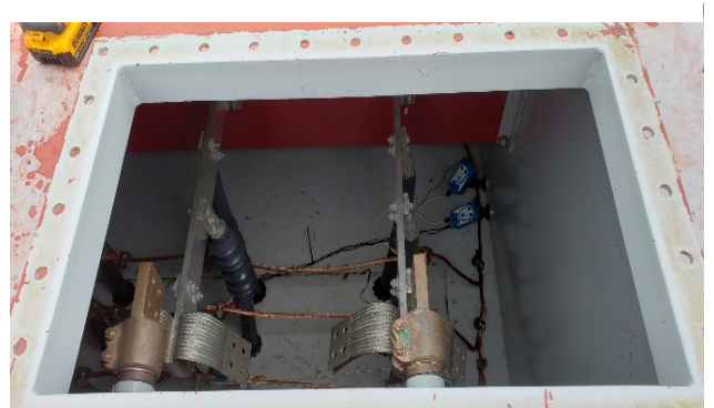
Figure 2 - IM500s installed inside the connection enclosure
