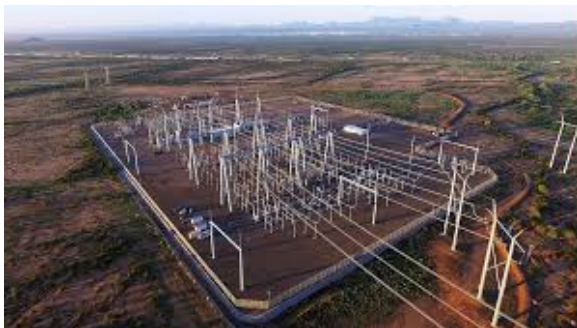
Figure 1. Remote Substation - TDWorld.com
