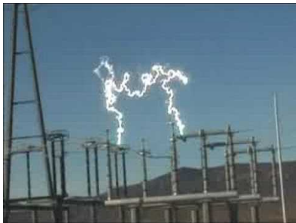
Figure 2. Arc Flash from a HV switch operation
